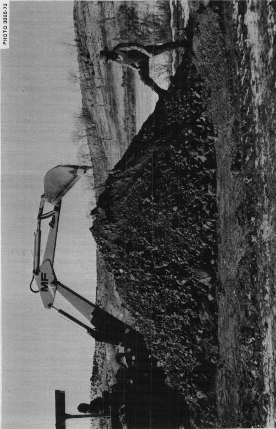
Fig. 3.1. Six and one-half feet of earth piled on December 1 over the 6-door Door-Covered Trench Shelter built by the manless family on November 24 and 25, 1973.
